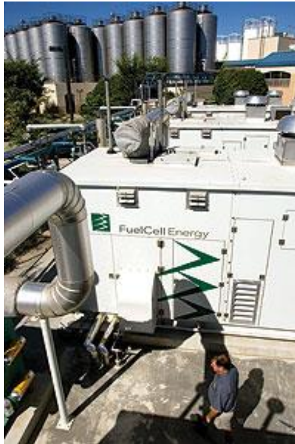
Figure 2. Four 250 kW hydrogen fuel cells units power a plant at Chico, California, with natural gas as a source of hydrogen.
