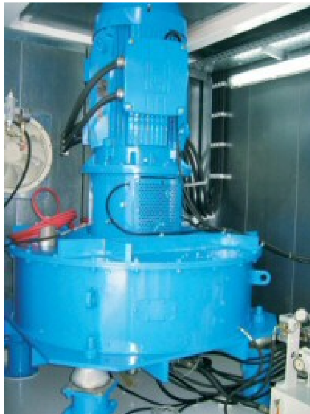
Figure 7. Enercon Flywheel. Source: Enercon.
