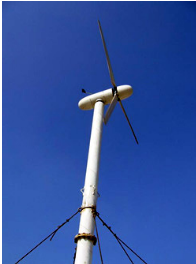
Figure 1. HGenerators 3.4 kW electricity and hydrogen producer wind turbine.
