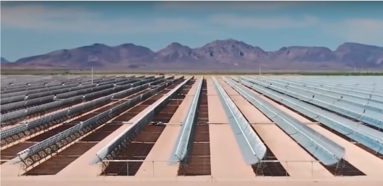
Figure 3. Concentrated Thermal Solar Parabolic Trough Power Plant.
