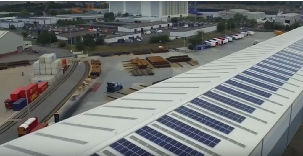
Figure 4. Commercial Roof Top Photovoltaic solar power Production.
