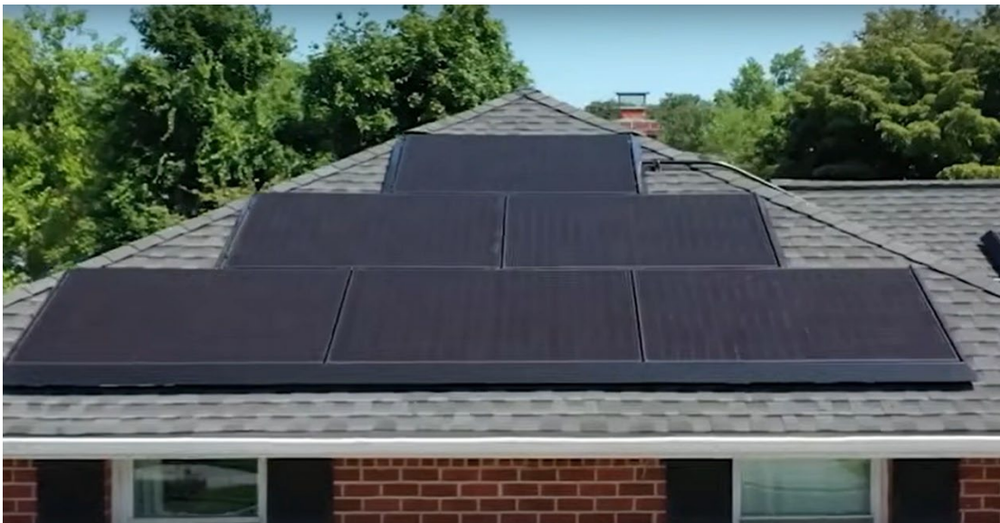
Figure 6. Domestic Roof Top photovoltaic solar panels.
