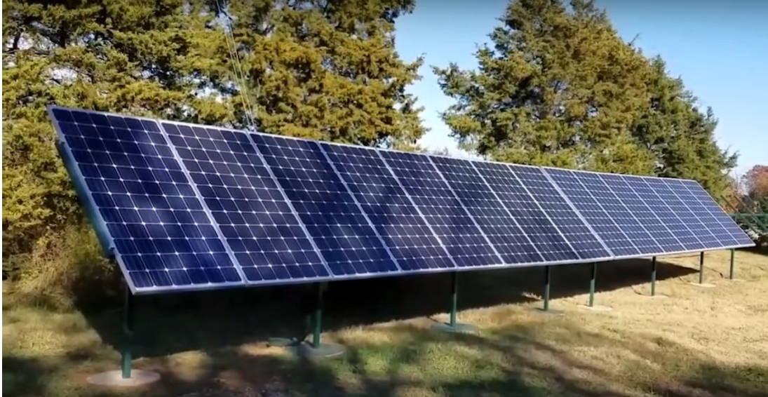
Figure 5. Domestic backyard photovoltaic solar panels.
