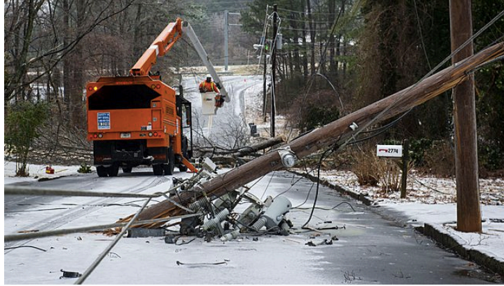
Figure 49. Downed overhead power lines, Doraville, Georgia, February 12, 2014.
