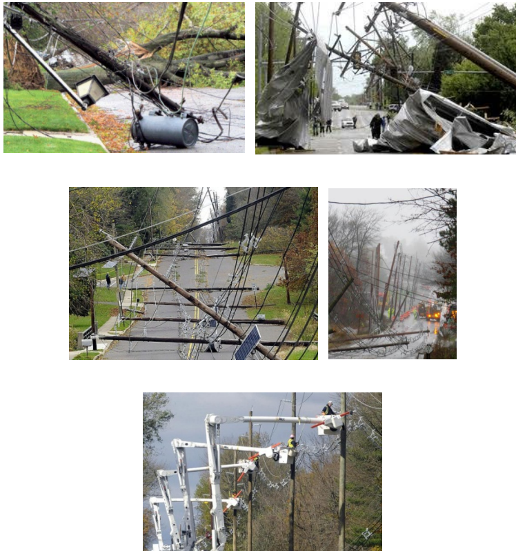
Figure 48. Repair crews from multiple states and utilities reportedly travelled from the West Coast to the East Coast of the USA to help restore the lost power from downed overhead power lines from Hurricane Sandy, October-November 2012.
