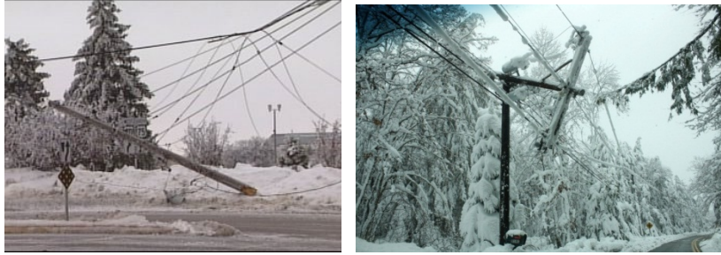
Figure 47. Downed overhead power lines caused by ice and snow storms.
