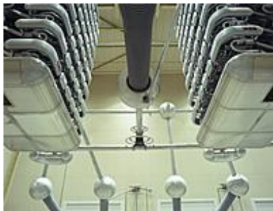
Figure 25. Huizhou valve hall, Three Gorges Guangdong Transmission, China. Source: ABB.
