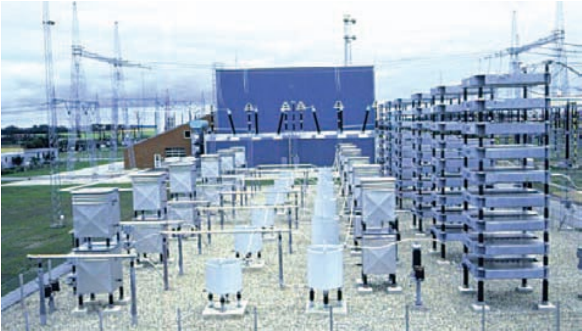
Figure 18. HVDC converter-station configuration. AC filters appear in the foreground, and the valve hall is in the background. Source: IEEE.
