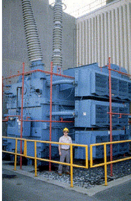
Figure 18. Damage to electrical transformers from the March 13, 1989 solar event.
