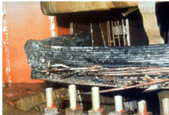
Figure 19. Transformer fire resulting from the March 13, 1989 solar event.
