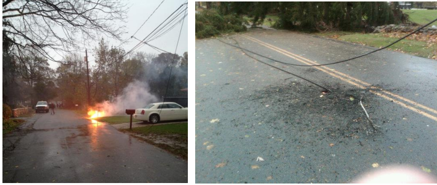
Figure 25. Downed overhead power lines constitute a sparking fire hazard in addition to their electrocution hazard.
