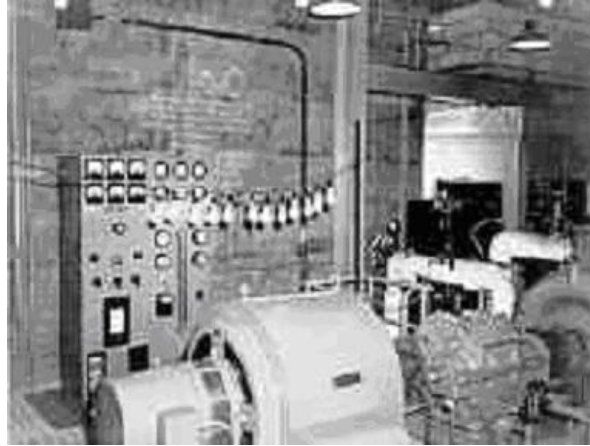
Figure 2. String of light bulbs was first nuclear-generated electricity from EBR-I on December 20, 1951.
