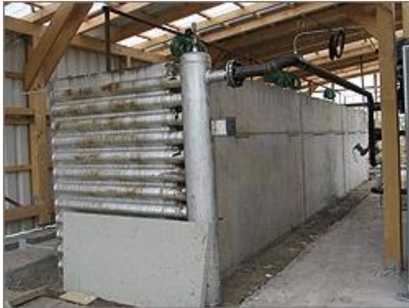
Figure 2. Concrete thermal energy storage unit.
