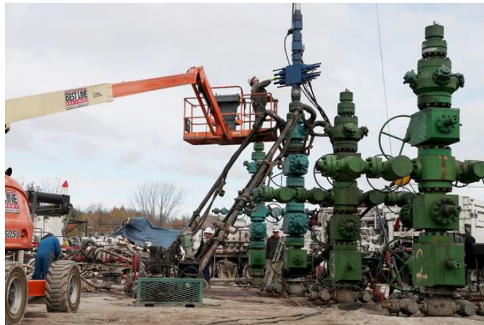
Figure 9. Blowout preventers (Christmas trees) at Marcellus shale formation, Camptown, Pennsylvania. Source: Southwestern Energy Co,
