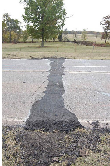
Figure 35. Highway 62 buckling caused by 5.7 magnitude tremor, Prague, Oklahoma, 2011 [12].
