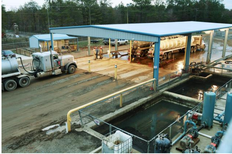
Figure 19. Water treatment plant for the separation of oil, sediment and antifreeze, Camptown, Pennsylvania, Marcellus formation. Source: Bloomberg.
