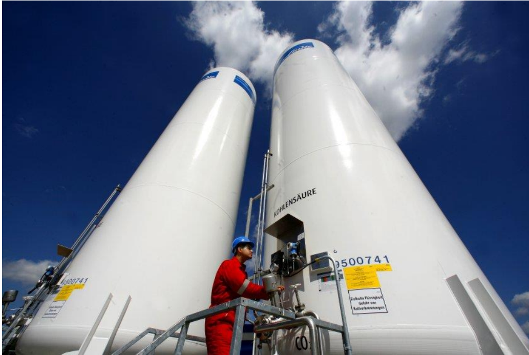
Figure 11. Carbon Capture and Storage, CCS of liquefied CO 2 demonstration plant at Ketzin, Germany. Source: ddp.
