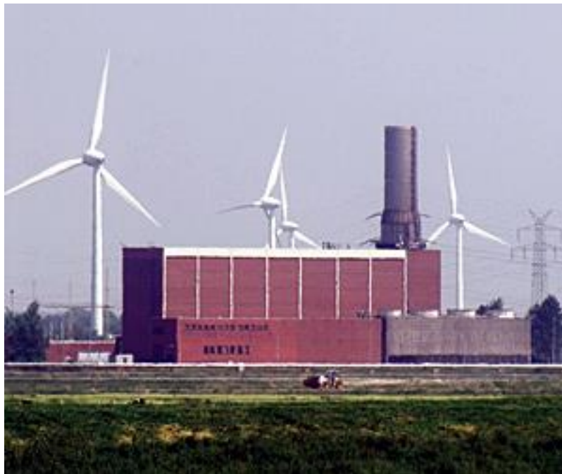
Figure 3. A 290 MW Compressed Air Energy Storage (CAES) in conjunction with wind power at Huntorf, Germany [2].
