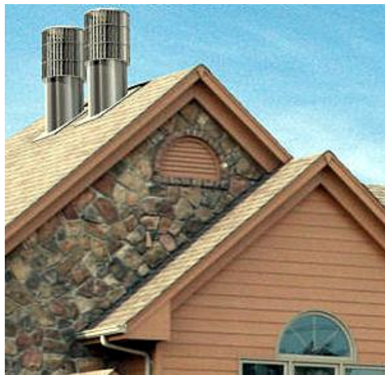
Figure 7. Roof-mounted vertical axis wind turbines.
