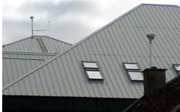
Figure 6. Roof wind turbines removed for repair.
