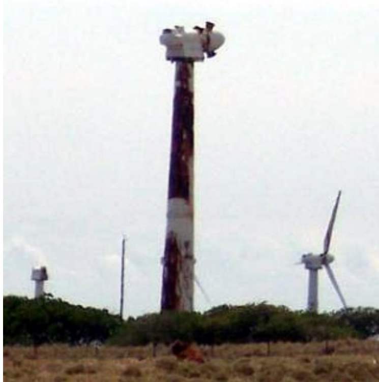
Figure 4. Abandoned and cannibalized Kamaoa wind farm turbines, Hawaii.
