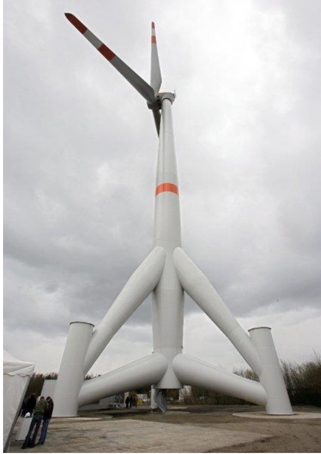
Figure 11. Prototype Multibrid M5000 offshore wind turbine with foundation.
