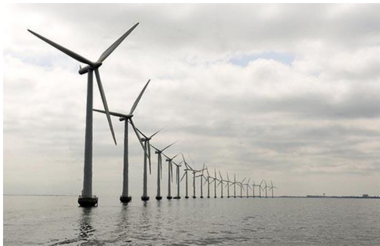
Figure 22. Offshore wind turbines. Source: GE.
