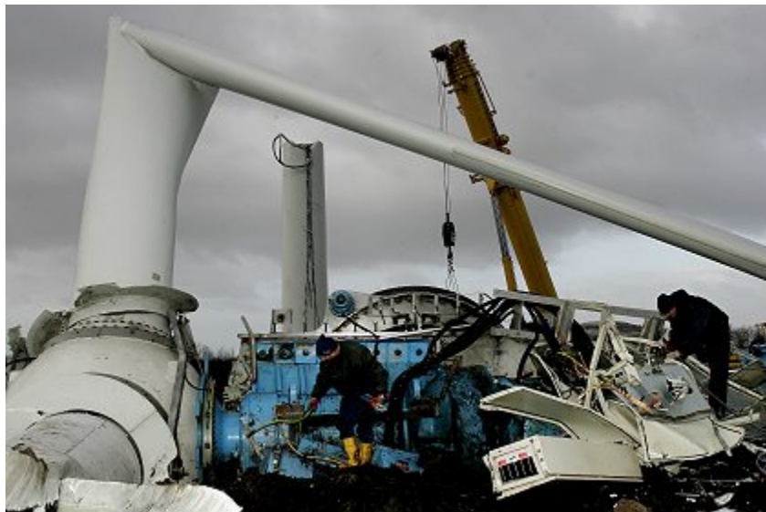
Fig. 1: Collapsed wind turbine in January 2007 in Germany. Source: AP.
