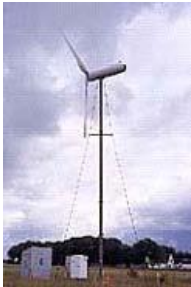
Figure 24. Guy wire poles for small wind turbines.
