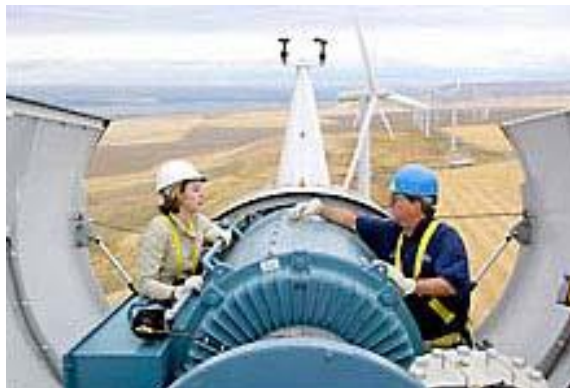
Figure 3. Open nacelle with two anemometers appearing in the back.
