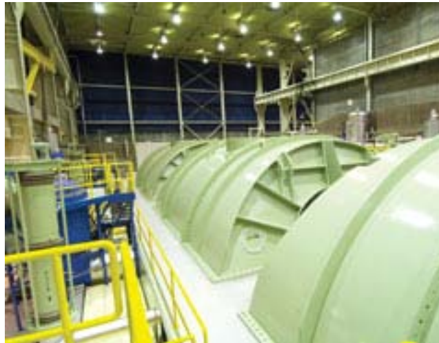
Figure 2. Browns Ferry BWR plant's turbine hall. Source: TVA.
