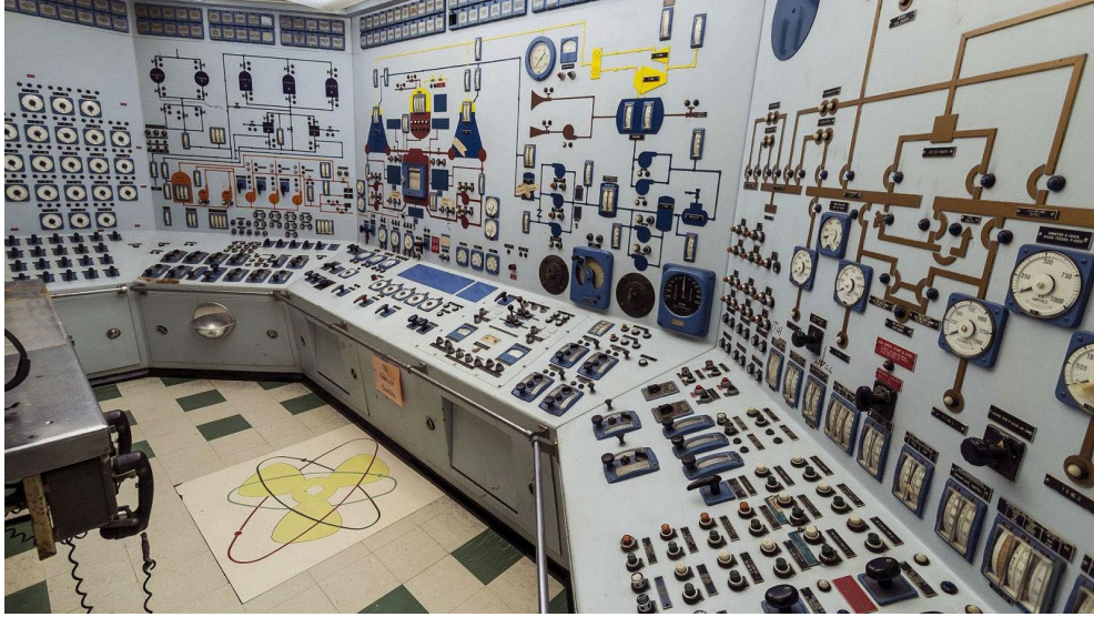
Figure 13. Control Room of the NS Savannah nuclear ship [10].
