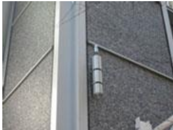
Figure 27. Area radiation monitor.
